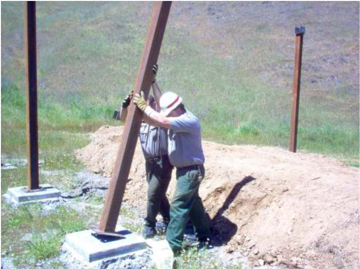
With both footings done, our friendly Rangers put up the post supports.
